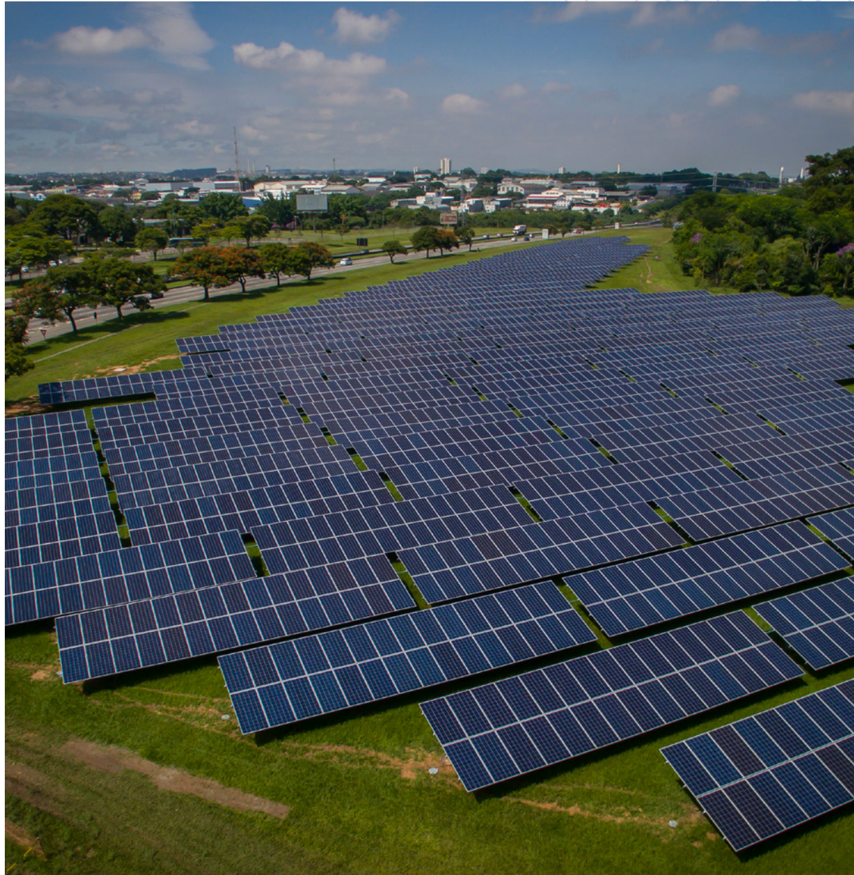
Solar panels help power Johnson & Johnson's São José dos Campos Campus in Brazil.
